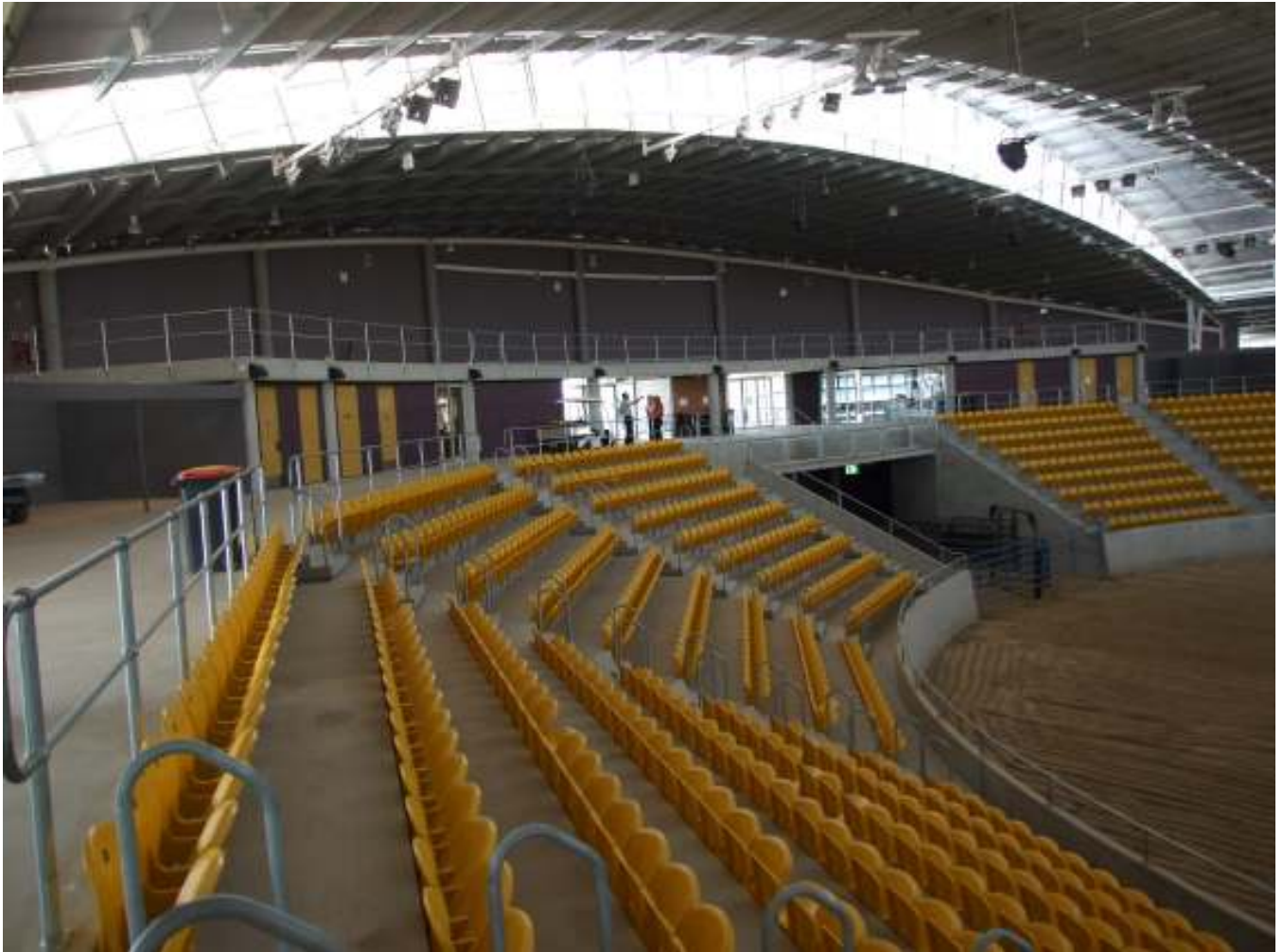
AELEC Stadium Seating Layout – Photo shows main arena entry doors in background
